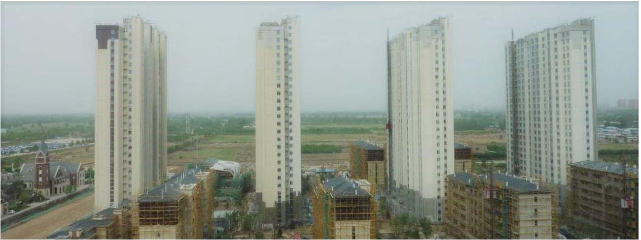
The construction site from a different perspective. After completion, the Bahnstadt Gaobeidian will be the largest Passive House settlement in the world. The apartments can be viewed during the Passive House Conference. © PHI
