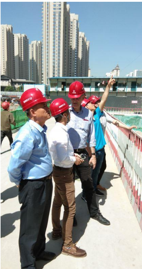
Passive House Institute staff members visit the Passive House construction site in the town of Taiyuan. The Conference in October will have the motto "Passive House worldwide" and will showcase projects from around the globe. © Passive House Institute
