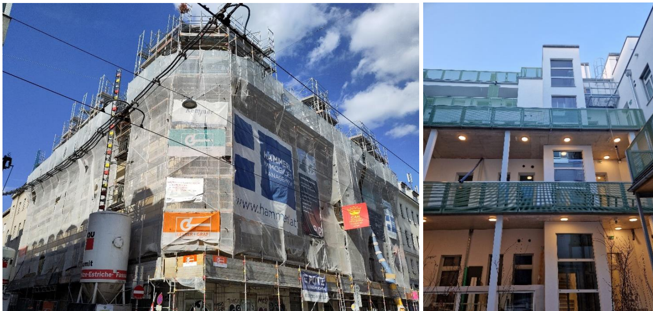
The 27 th International Passive House Conference in Innsbruck will focus on EnerPHit renovations: The modernisation of this Wilhelminian style building in Vienna using Passive House components is almost complete. © Schöberl & Pöll
