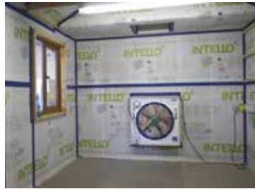
Figure 93: Airtight room, light weight construction and including a windtight / humidity resistant external membrane. © MosArt
